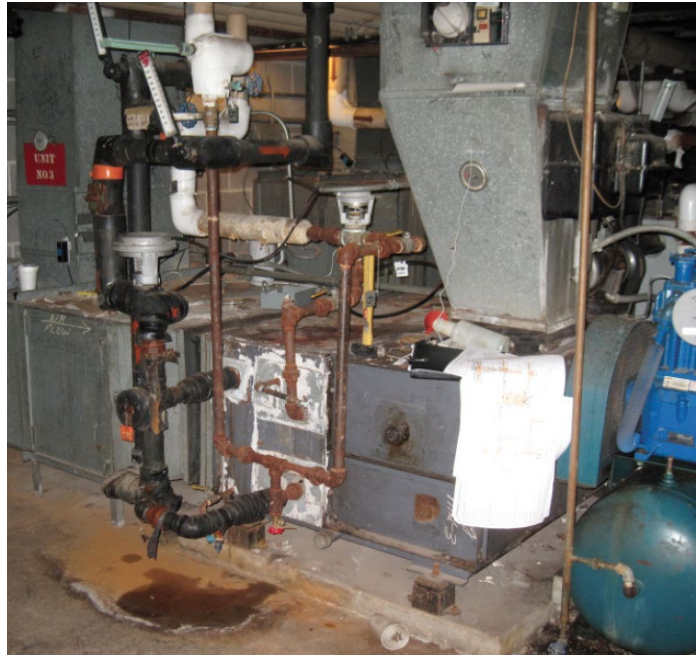
Nursing home return air handlers require replacement.
